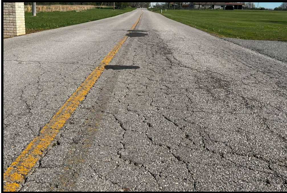
11: Bausinger Road. Signs of Pavement distresses.
