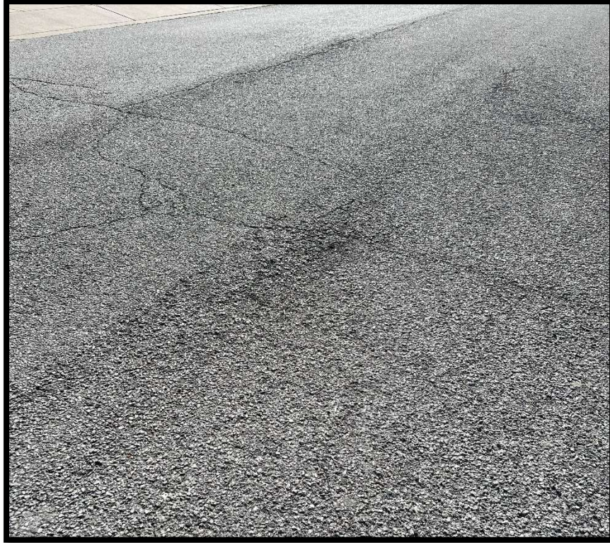
9: Penzo Ave. Signs of Pavement distresses and raveling.
