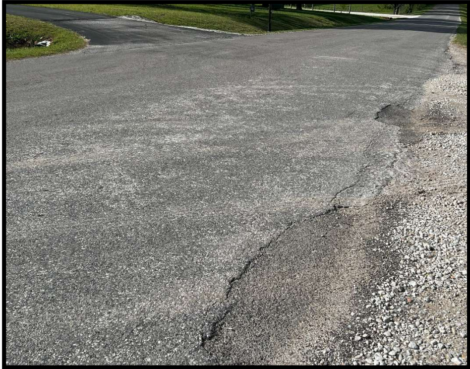
5: N Pianalto Road. Signs of Pavement edge distress and raveling.
