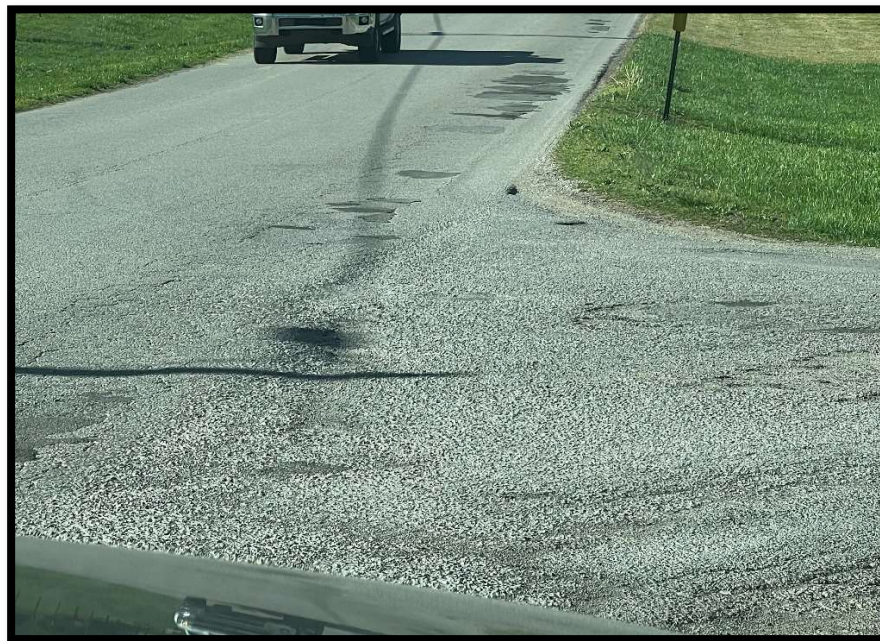
4: Liberty Ave and N Barrington. Signs of Pavement distresses and failures.
