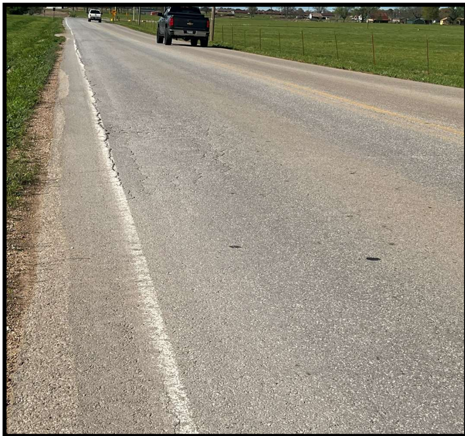
14: Dowell Road. Localized pavement distresses and raveling.
