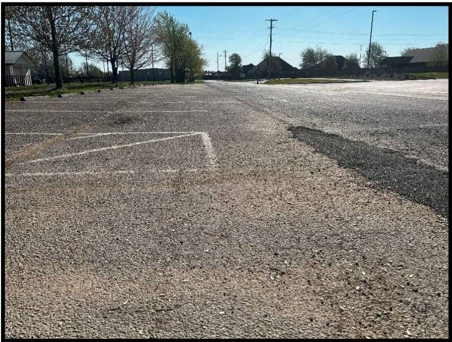
6: E Bandini Parking. Signs of Pavement distresses and failure.
