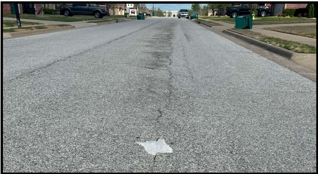
8: Ranalli Ave. Signs of Pavement distresses and raveling.
