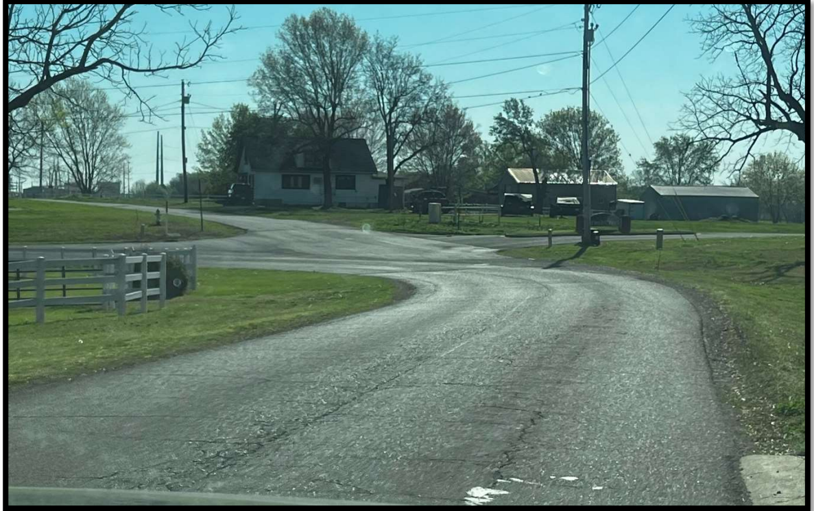
1: Liberty Ave, west of Brush Creek Road. Signs of Pavement distress and cracking.
