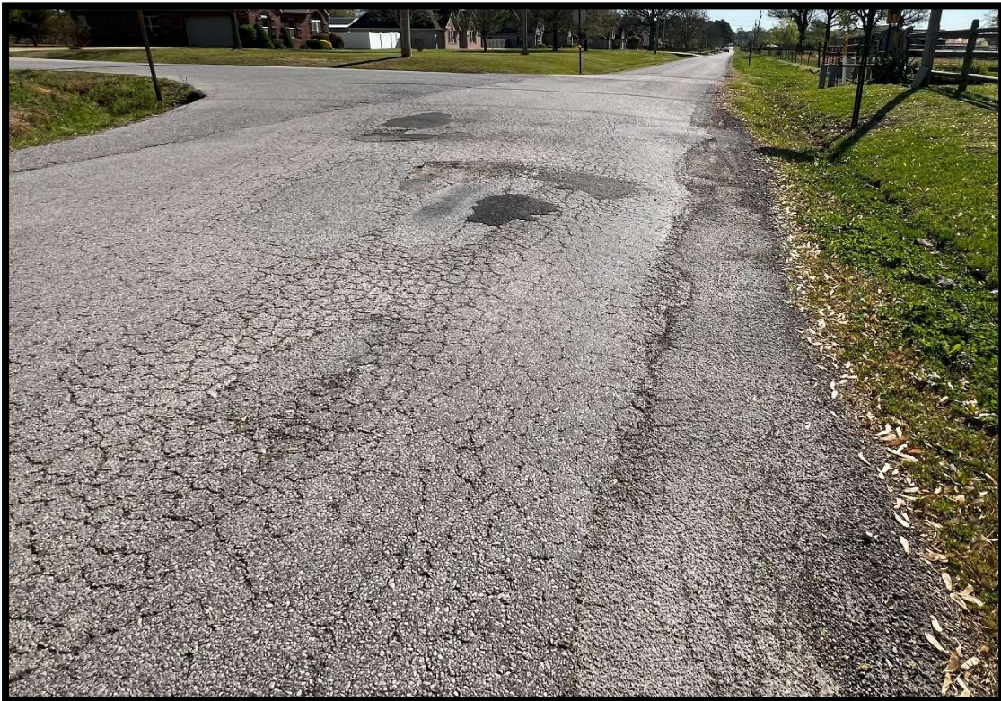
10: Morsani Ave at S Mantegani Road. Signs of Pavement distresses and failure.
