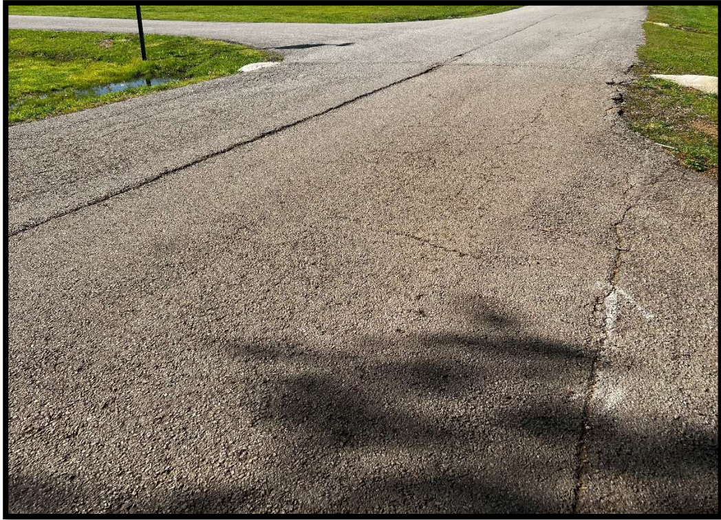
7: Cortiana Street. Signs of Pavement distresses.
