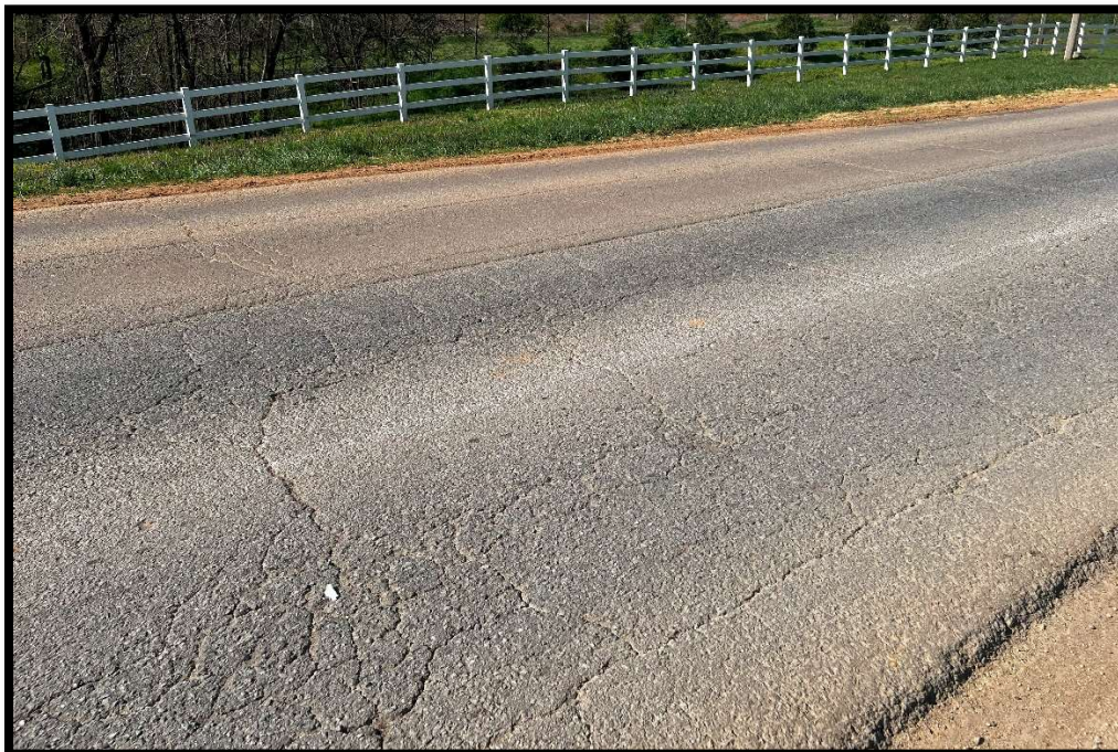
12: Arbor Acres Ave, near Dowell Road. Signs of Pavement distresses.
