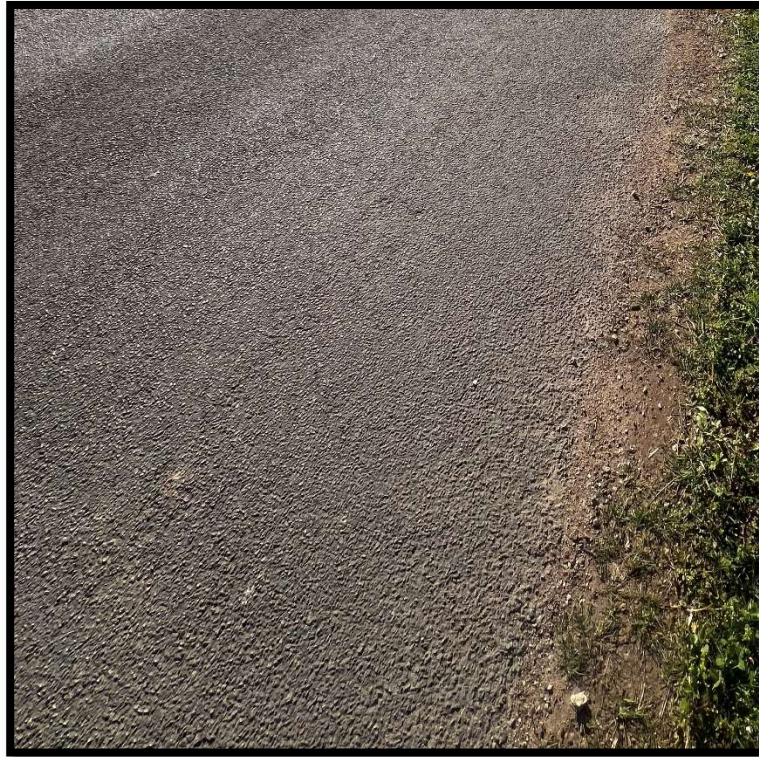
3: Liberty Ave, near Foster Lane. Signs of raveling.
