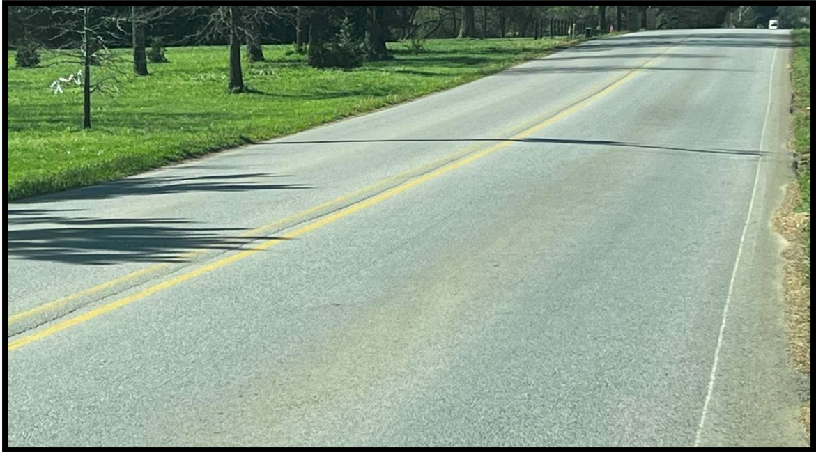
13: Klenc Road. Fair Condition with early signs of raveling.
